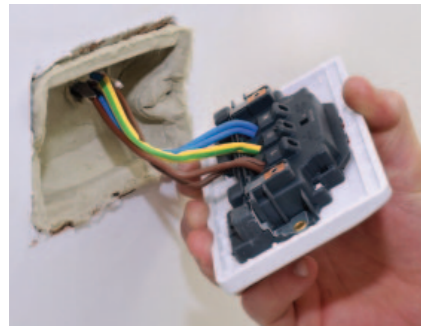
This power outlet in a party wall has an 'intumescent' seal that expands to block the opening in the event of fire
