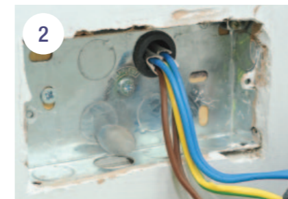
Wood behind the switch box
